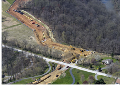
The Atlantic Sunrise gas pipeline is bored under Main Street west of Conowingo. In this aerial photo taken April 18, 2018. RICHARD HERTZLER | Staff Photographer
